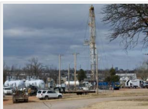
Contractors work with New Dominion to recomplete a well in the company's south Oklahoma City field. (Courtesy Photo)
